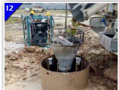
12 After Completing Casting, Tremie Pipe And Temporary Casing Are Withdrawn. The Casted Bored Pile Location Is Suitably Protected For Safety.
