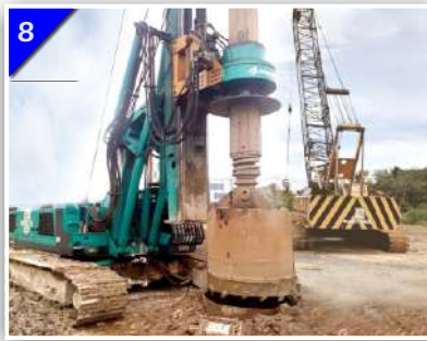
8 When Rock Is Encountered, Using Rock Coring Tools To Bore Through To The Required Rock Socket Depth.
