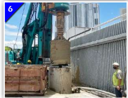
6 When Steel Casing Reached Intended Depth, Boring Of The Hole Continues Until The Designed Depth Of The Pile.
