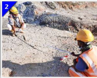
2 OffSets From The Pile Position Are Marked As Guide For Later Reference To Pile Point.
