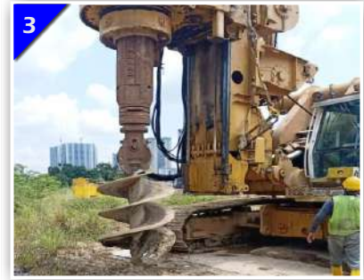
3 The Drilling Rig Is Moved To Near The Pile Position. The Kelly Bar Is Mounted With An Auger And Placed Directly Above The Pile Point. By Means Of Spirit Level The Kelly Bar Is Checked And Adjusted For Verticality.
