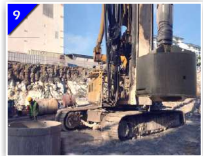
9 The Bored Hole Is Cleaned With Cleaning Bucket. The Final Bored Depth Is Checked And Measured Together With The Supervising Engineer's Representative.
