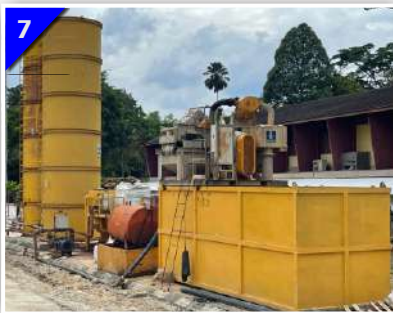
7 Soil Stabilization Fluid Plant Set Up At Project Site. Besides Water, Special Fluids (Bentonite Or Polymer) Are Specifically Mixed And Pumped Into Bored Holes During Boring Works To Stabilize The Soil.
