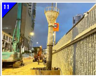
11 Tremie Pipe Is Installed For Full Depth Of Hole. Concrete Is Placed Through Tremie Pipe Until Beyond The Designed Cut Off Level To Ensure Entire Pile Is Casted With Good Quality Concrete.
