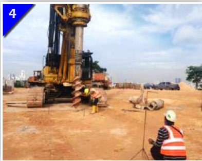
4 The Auger Is Placed Directly On The Pile Point. With Slow Speed And Repeated Shallow Penetration Into The Soil A Hole Is Formed. The Shallow Augered Hole Is Checked For Accuracy Of Pile Position.
