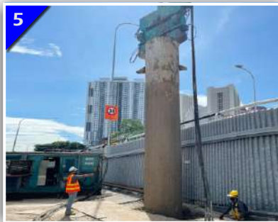
5 Temporary Mild Steel Casing Is Then Installed To Provide Stability Of The Bored Hole. The Verticality And Position Of Casing Is Constantly Checked To Comply Designed Position Of Pile.
